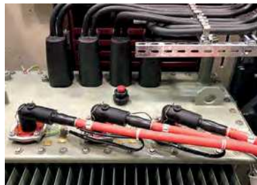
Transformer connection with 200LR
