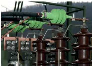
AFN10 as a transformer connection
