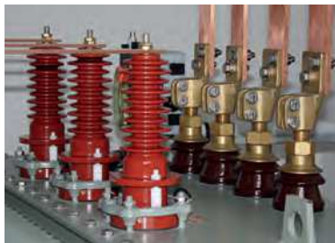
PITO-E on transformer with bushings
