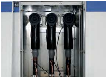
SF-6 system connection with 480TB
