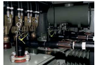
Transformer connection with 158LR
